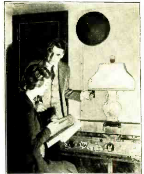
A typical room installation in the New Yorker Hotel. The wall plate under the man's hand contains the four-station selector switch and volume control; the reproducer cone is above it.
